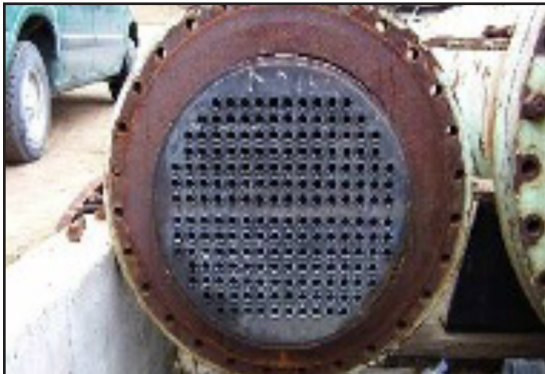
Corroded tube sheet
